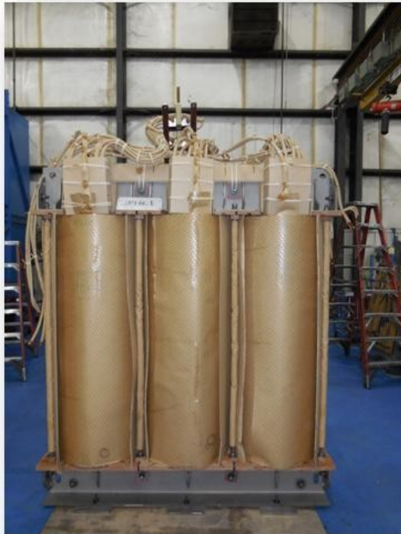
Rebuilt Core/Coil Assembly
